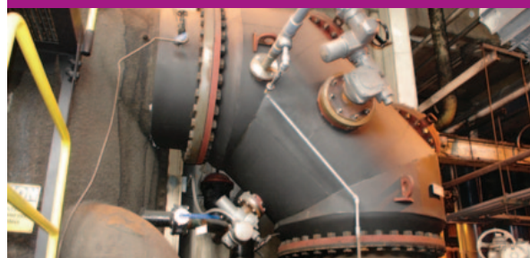
Debris filter installed
