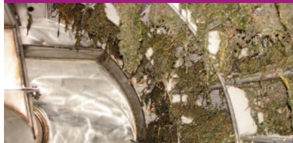
Inside debris filter prior to cleaning cycle
