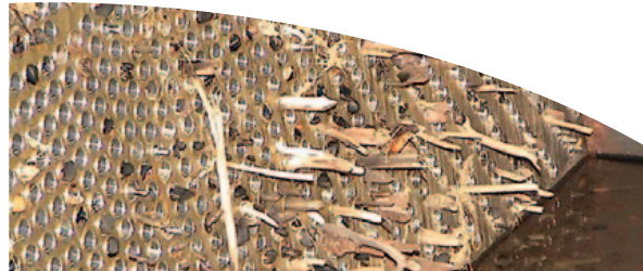
Condenser tubes without debris filter
