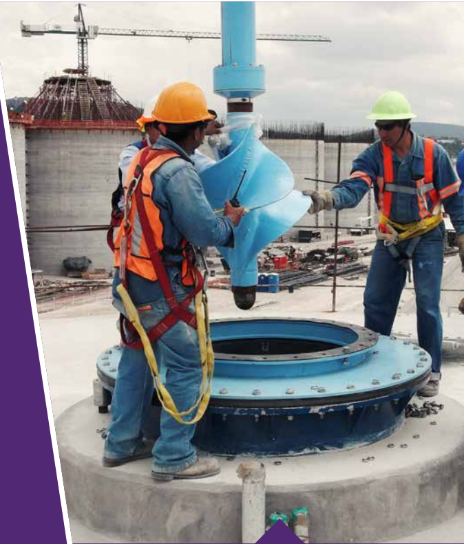
ATOTONILCO PTAR, MEXICO: (1) RDT-T-75-36 with over 60' long Draft tubes.
