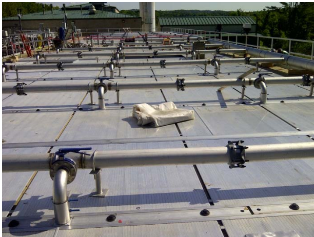
Airbeam Cover Aeration System
