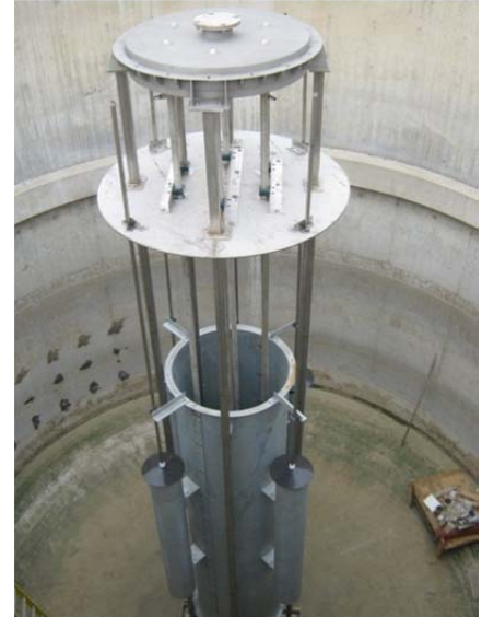
MEDT Aeration Equipment Under the Airbeam® Cover
