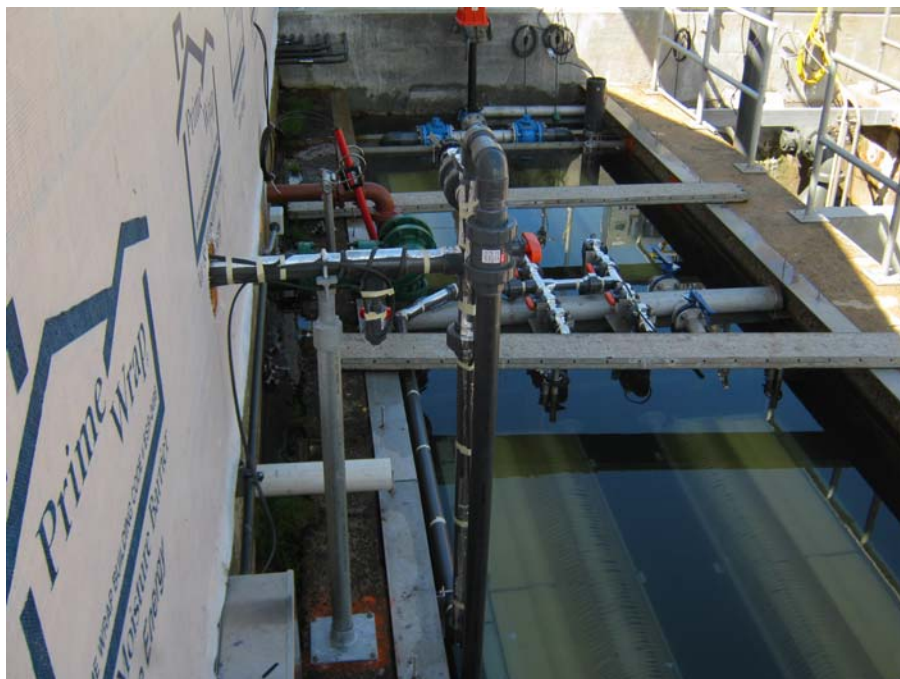
Membrane Thickening Tank at Patchogue WWTP
